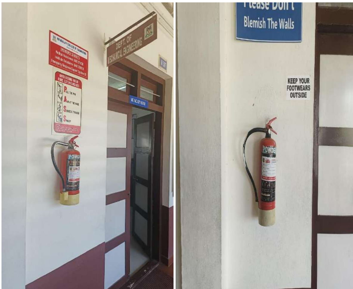
Fire suppression extinguishers
