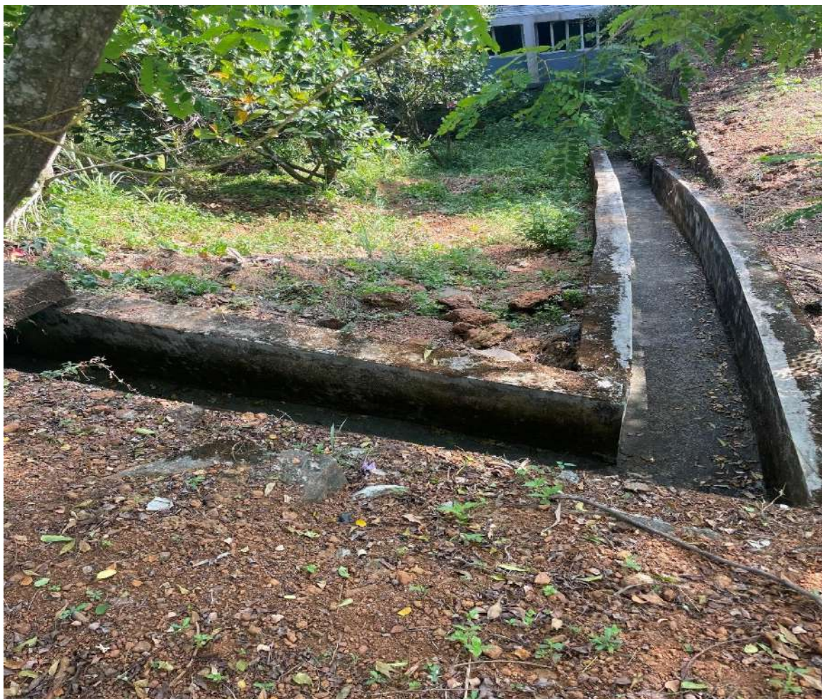
Open Rain water channels
