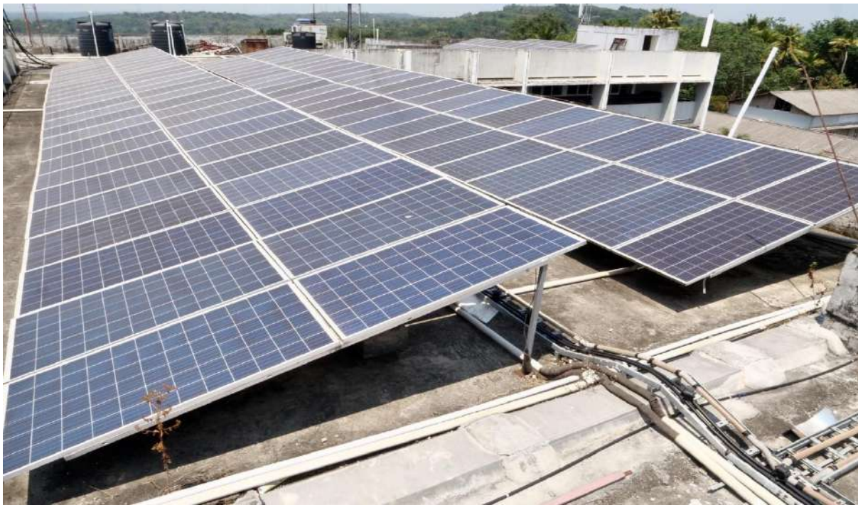
Solar panels on roof top
