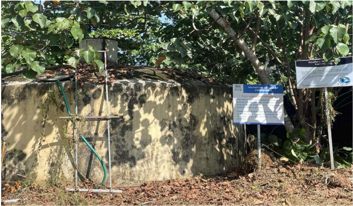
Rain water Collecting Tank (1 lakh )
